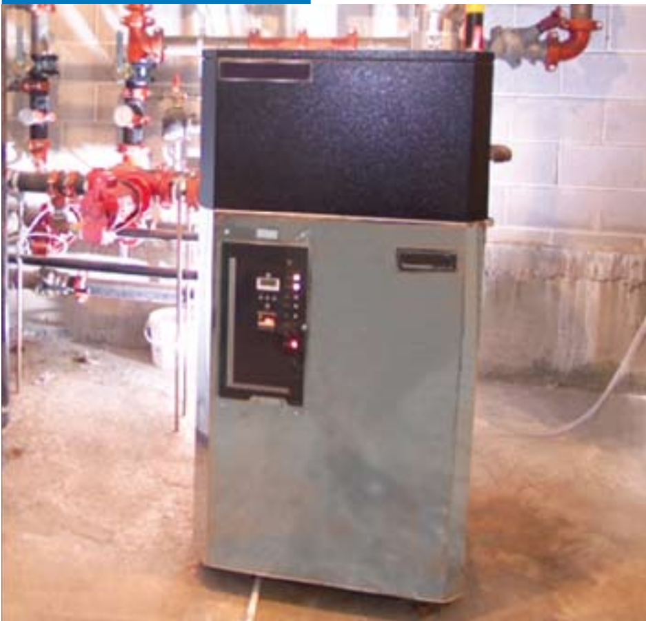
The newly installed, 95 percent efficient high condensing boiler at 1035 Powers Street.
