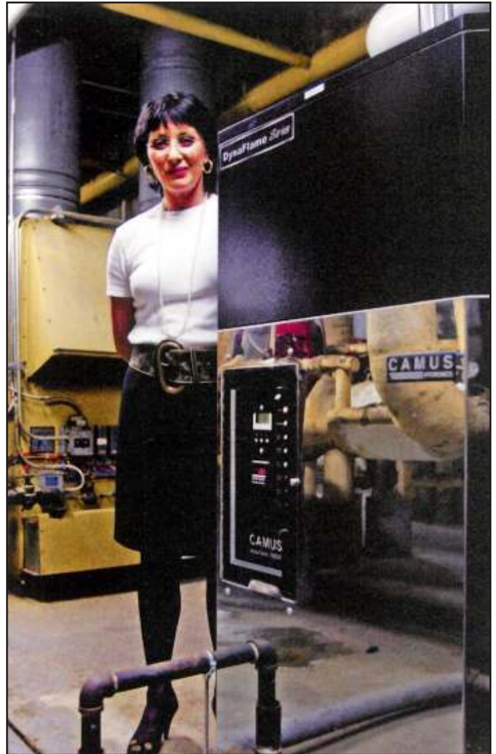
Elizabeth Beaudin, property manager of Lexington Condominiums on Carlton St., shows off the building's new CAMUS boilers. The condo might have done more energy upgrading on site, but the Condominium Act restricts the access to reserve funds.
